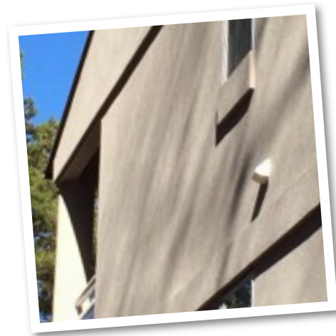
This clothes dryer duct - above- was installed in one of the newly constructed end walls -with no Board knowledge or approval. Owners are responsible for repairing any common area property which they have damaged.
