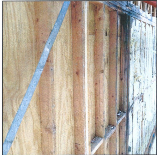
View of eastern portion of the north wall. This wall has been historically repaired at all three floors. Note that the wall insulation was not found to exist. New wall insulation will be installed.
