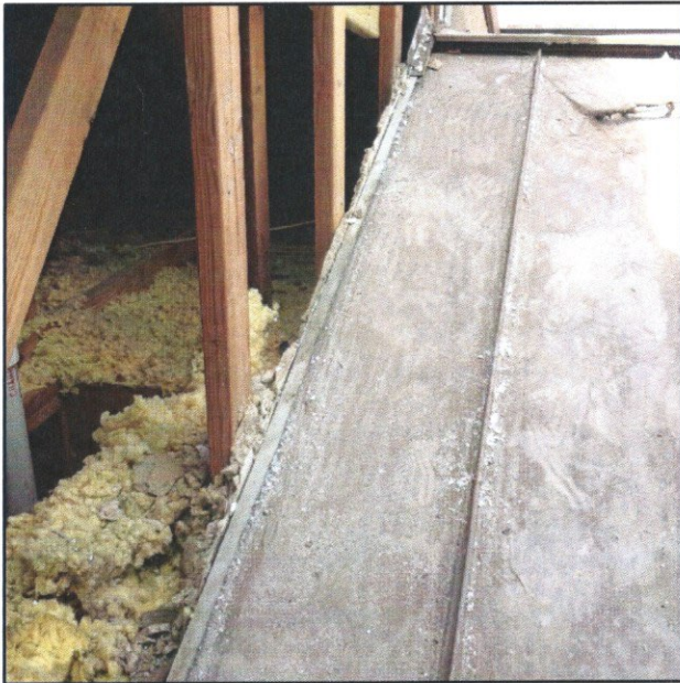
Views of roof to attic wall intersection. A new flashing detail will be developed to repair this area.
