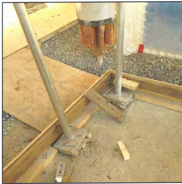
View showing wood edge forms and temporary wood walkway for Unit 101 access.
