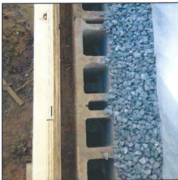
View showing wood edge forms and existing concrete masonry wall prepared to receive new concrete.
